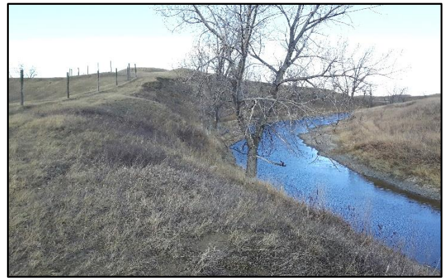
Looking northeast at standing water adjacent to former irrigation canal embankment
