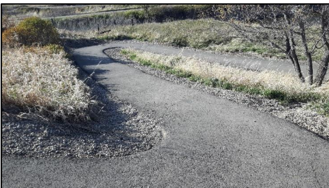
Looking at steep switchback area within outer trail loop
