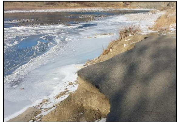
Sloughing adjacent to trail at Pavan Park (Lethbridge, AB)
